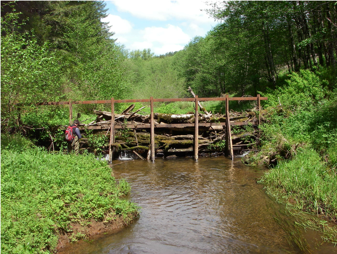
Photo 23. Un-maintained trash rack above HWY 26. Mainstem Rock.
