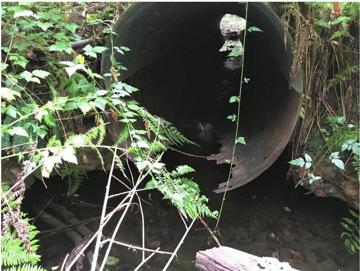
Photo 137 Trib A (Sally) Failing Culvert
