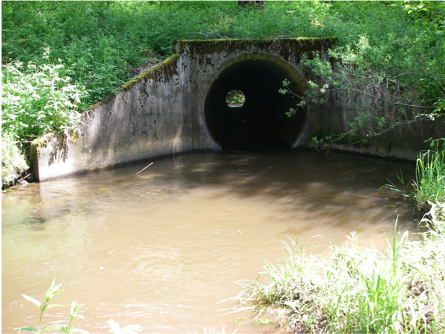
Photo 33. Under-sized HWY 26 culvert in Rock Cr Anchor Site 9. Compromising resource migration and delivery to lower mainstem Rock Cr.
