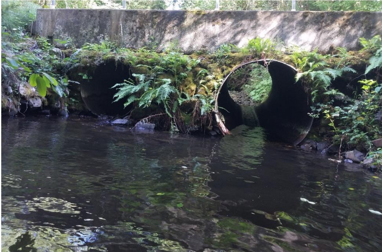
Photo 133 Little Rackheap Failing Culverts
