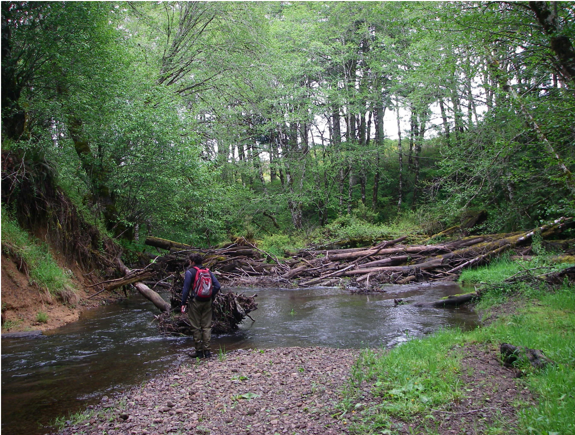
Photo 32. Large full-spanning jam formed on collapsed log stringer bridge still holding Rock Cr Anchor Site 8 together.
