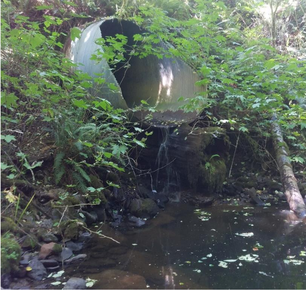
Photo 17 Perched Culvert, 5ft
